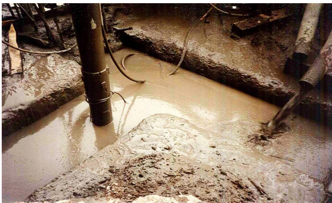
Photo 10: Airlift pipe for de-sanding and bottom cleaning.
