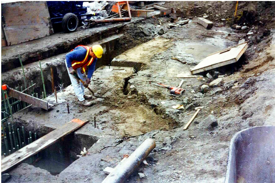
Photo 2: Failure of guidewall due to discontinuation of steel reinforcement at joint.
