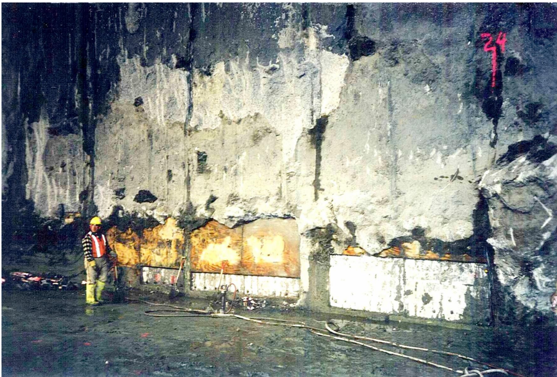
Photo 21: Exposed plywood and Styrofoam ready for removal from keyway. Significant overpour above keyway.
