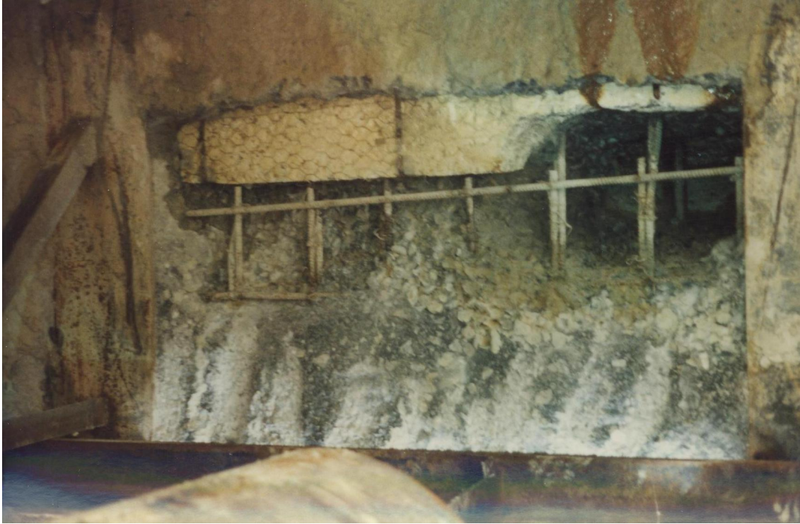
Photo 22: Void in slurry wall at keyway location.
